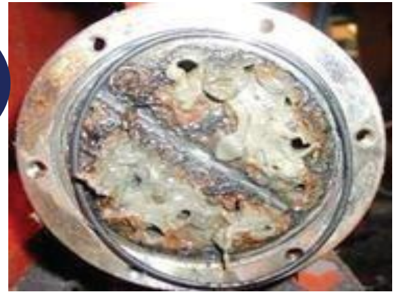
Scale inside condenser
