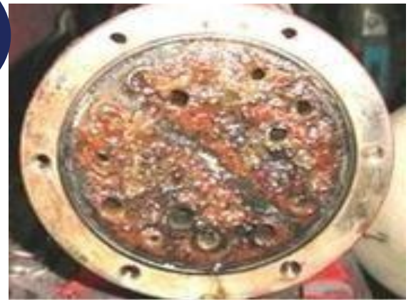
After installing Scale Doctor, cleaner condenser
