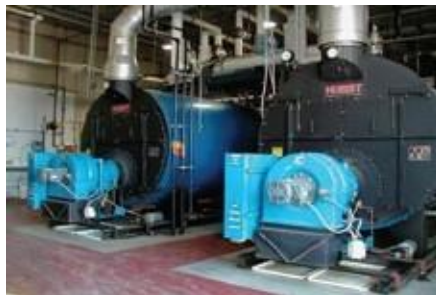
Boiler and condenser
